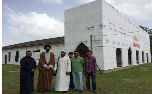
H.I. Syed Sulayman Abidi (HA) visits construction site of Masjid Al-Rasul No. 2 a.k.a. Fifth Ward Mosque
